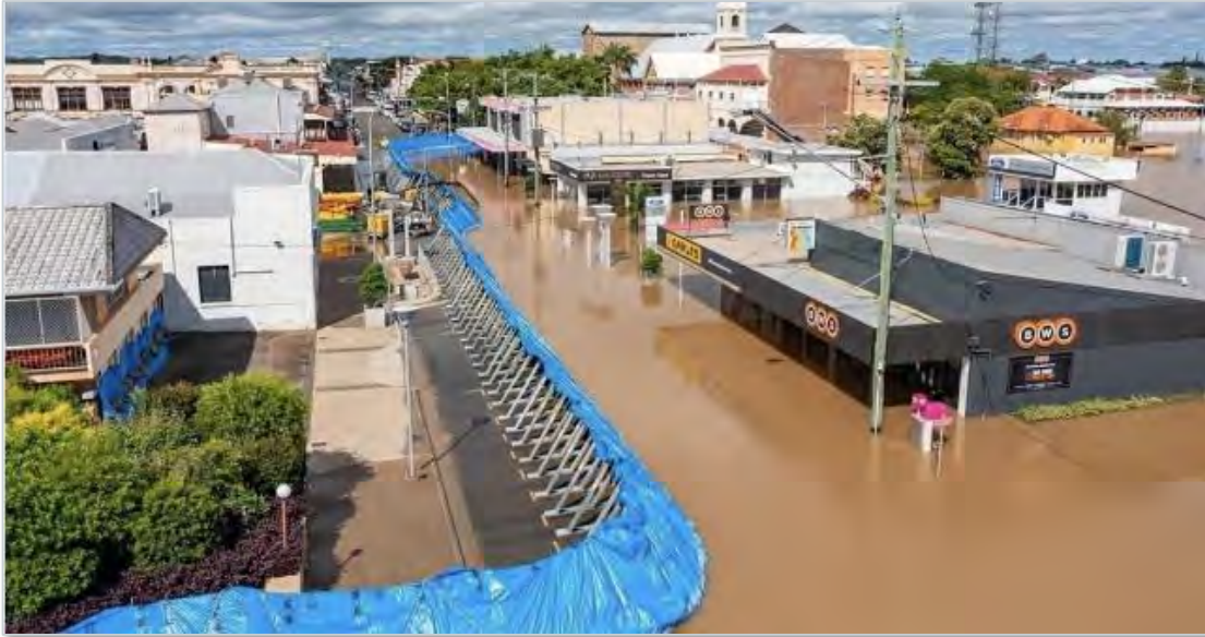
Figure 29 - Inflatable temporary flood barrier
