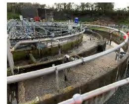
Westport WWTP Bioreactor
