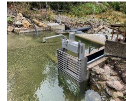
Intake Gate and Screen
