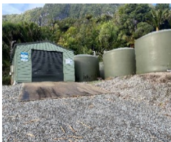
Punakaiki WTP Overview
