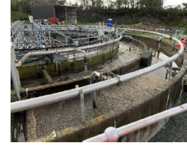
Westport WWTP Bioreactor
