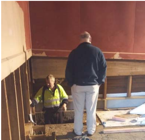
Theatre Storeroom – preparation of a corner foundation footing prior to reinforced concrete pour.
