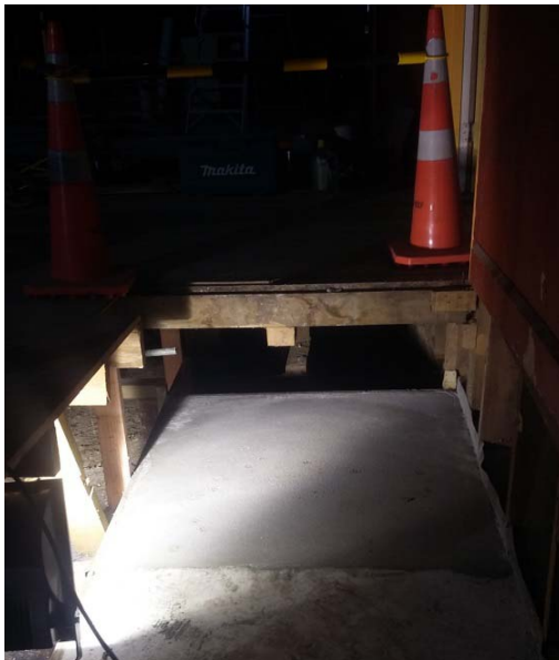
Theatre Ticketroom – corner reinforced concrete foundation footing prior to installation of portal steel post.
